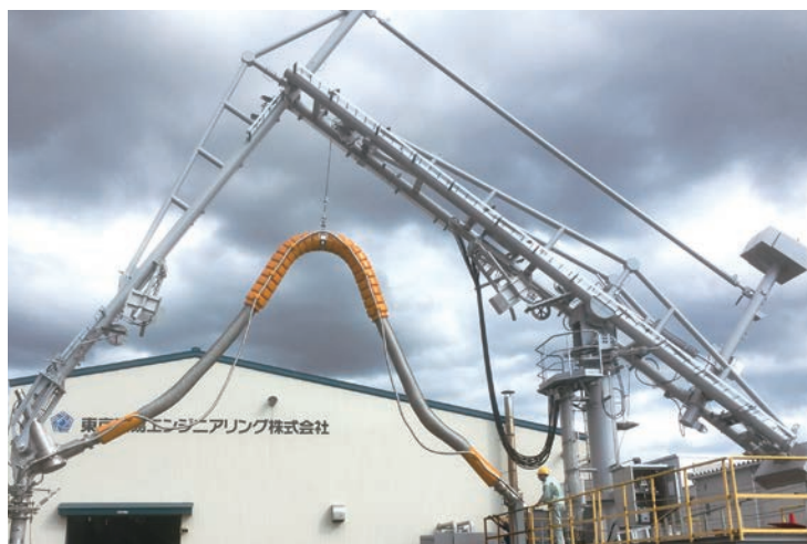
Fig. 6 Loading arm systems for demonstration project
