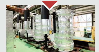
The boiler is then fitted with sensors and "clothed" with insulation sheets. This is the semi-final stage of boiler construction.
