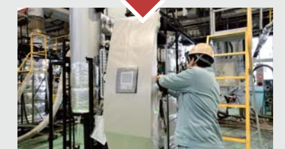
Finally, a cover casing is installed. The door's front panel is equipped with a controller used for remote monitoring of the boiler via communication lines.
