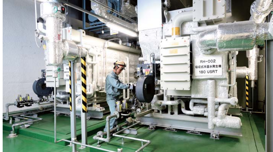
The Efficio absorption chiller-heater in operation at Osaka Medical College Hospital. Two Efficio units cool and heat the entire Surgery Building. With dual lines—one dedicated to cooling and another to heating—the hospital can control both temperature and humidity to optimize the surgical environment of each operating room according to its needs.
