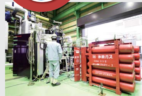
A hydrogen-fired once-through boiler used for the verification testing. The red tank contains the hydrogen.
