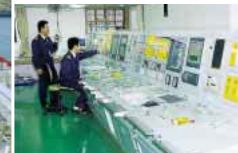
The cargo control room on board the ship is equipped with an integrated monitoring and control system (IMCS) developed by Kawasaki. It enables monitoring and control of cargo handling operations as well as monitoring engine conditions.
