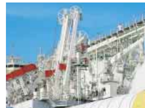
Unloading arm. LNG is discharged through these pipes.
