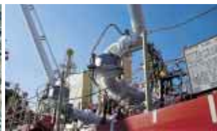
The loading arm is completely frosted over due to the cryogenic temperature.
